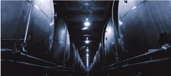
Fill level measurement in tanks
